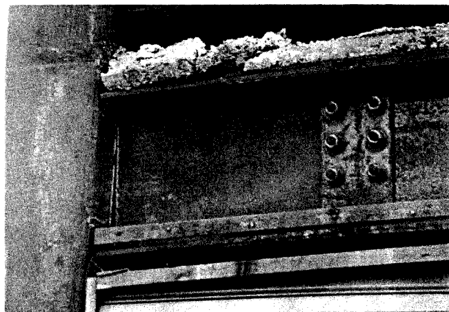
Fig. 20. Failure of the beam-to-column welded connection at the first storey of the building shown in Fig. 7.
